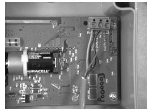
Figure 2. Terminal Block Connection
